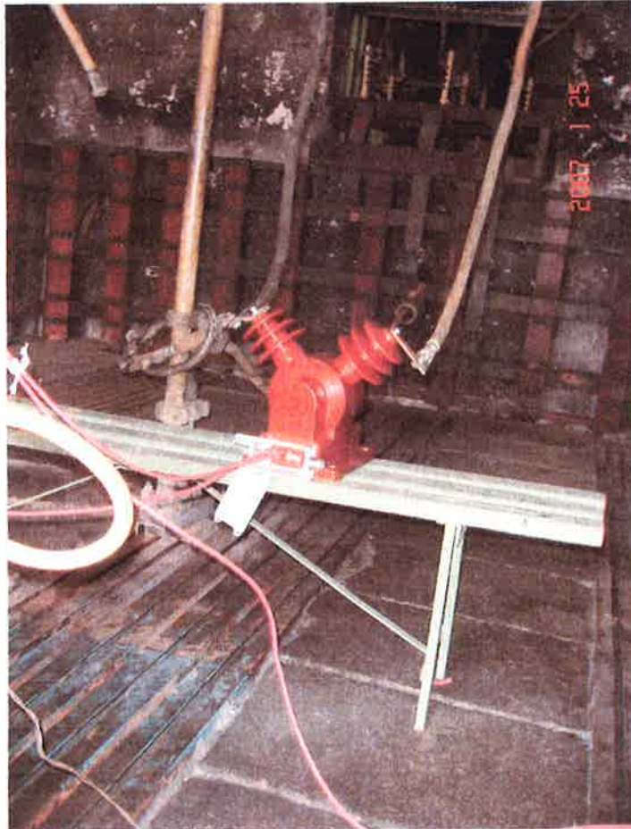
Photo – Aspect of the voltage transformer in the testing circuit
